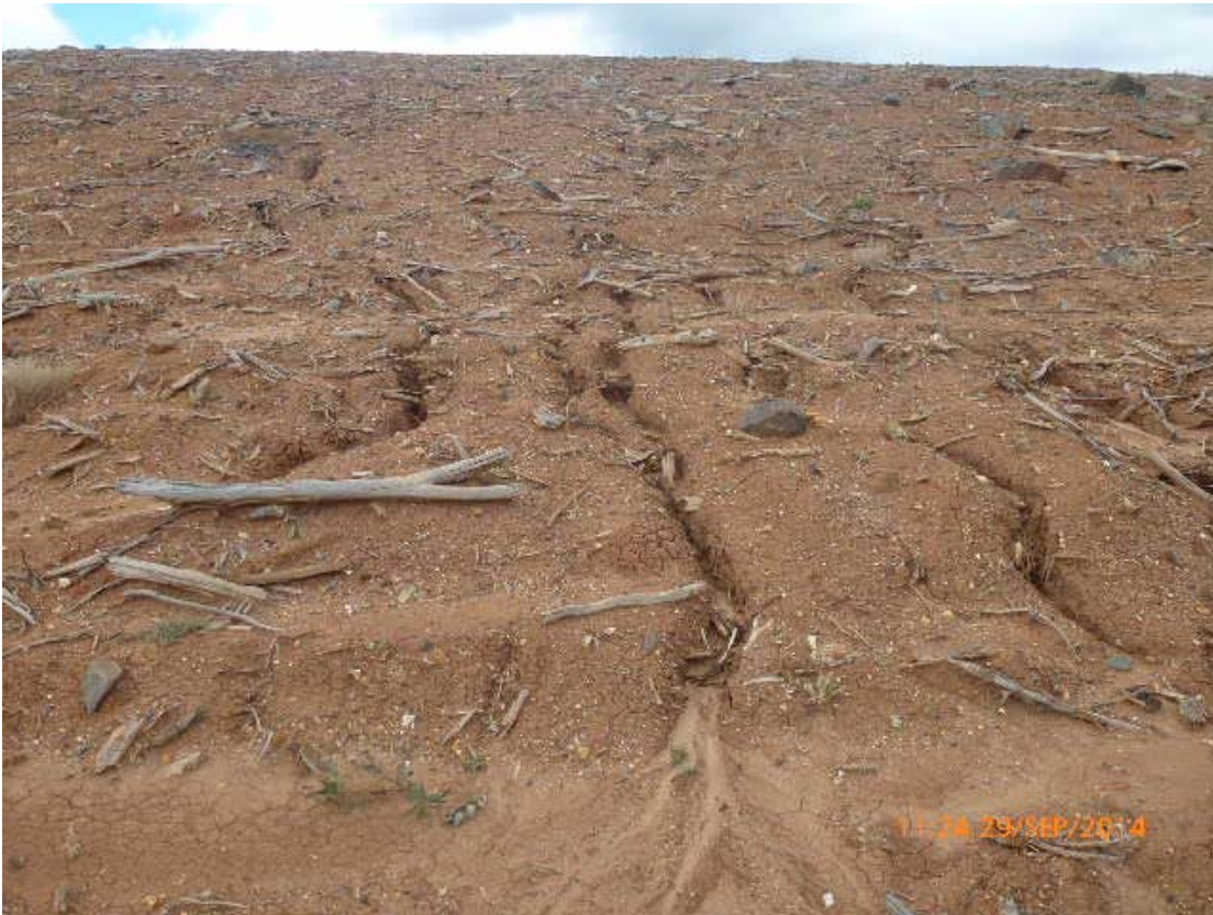
Plate 5.2: Unsatisfactory utilisation of vegetation debris providing insufficient surface cover
